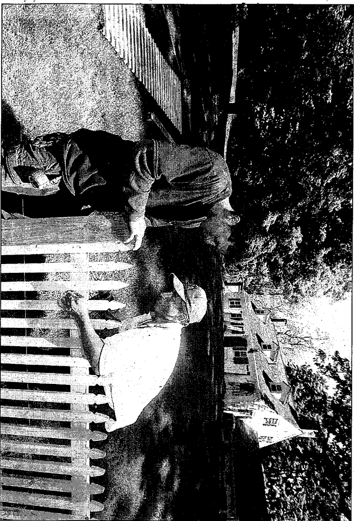
Carlos Bonilla, left, and Victor Mata of the Artistic Fence Company work to replace a 250-foot-long fence in front of the historic Luke Miller House in Madison on Friday. The old fence had stood since the 1950s and was a replica of the first fence built on the property in 1894.
